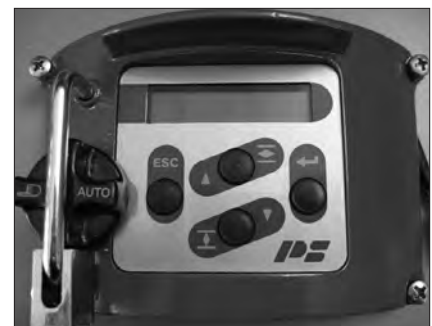
PSC.2 Local Control
